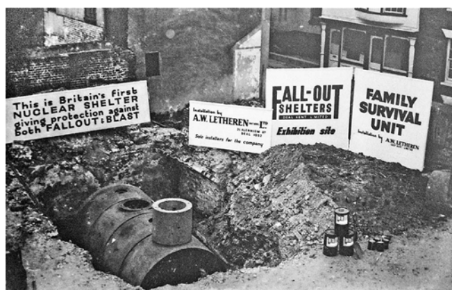
The shelter being installed on the site of the Royal Oak pub. Photo Basil Kidd
